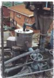
KC-CD12SS (Stainless Steel) at work in Avgold's Fairview Mine.
