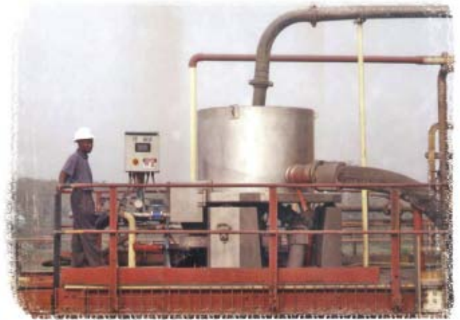
A custom manufactured stainless steel KC-CD30 in operation at AngloGold Ashanti – Biox Plant Obuasi, Ghana.
